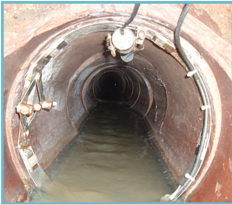
Flow monitoring device
