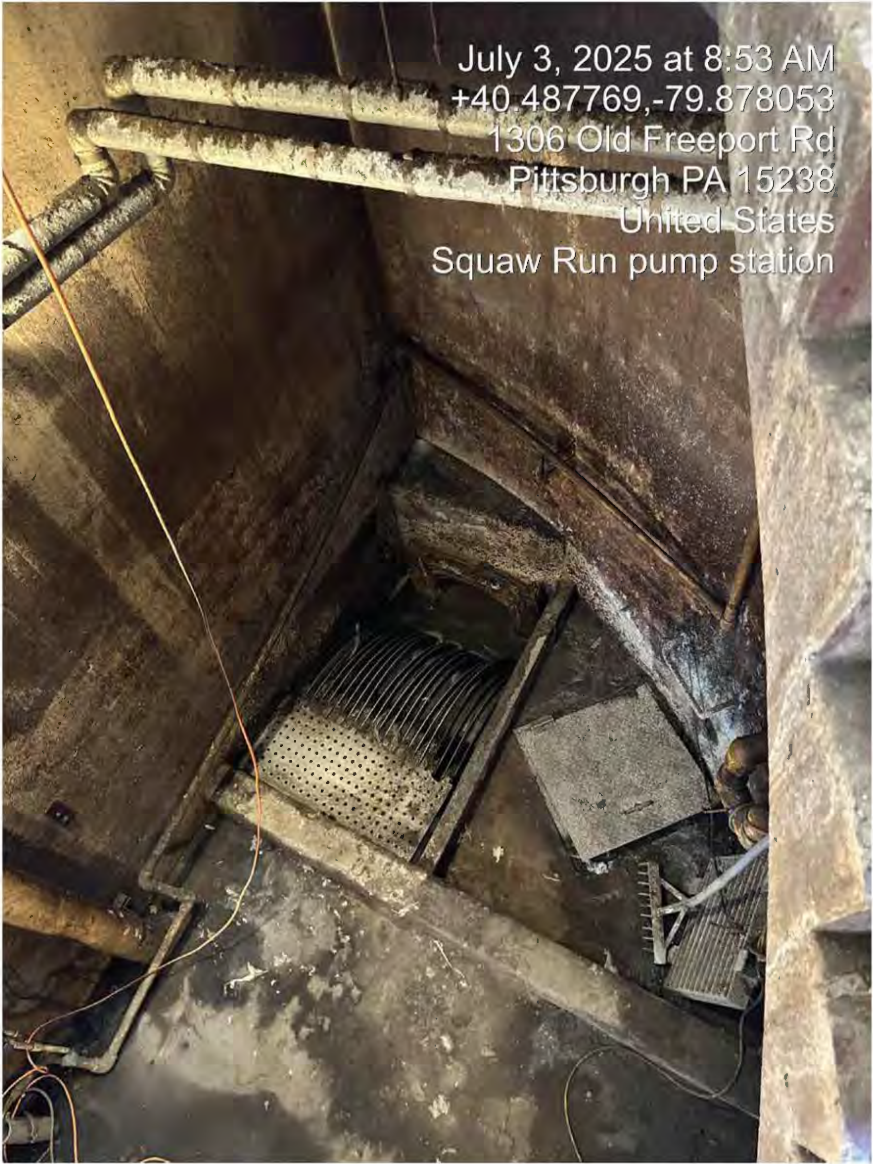
BYPASS PUMP DISCHARGE TO EXISTING PUMP STATION INFLUENT BAR RACK
