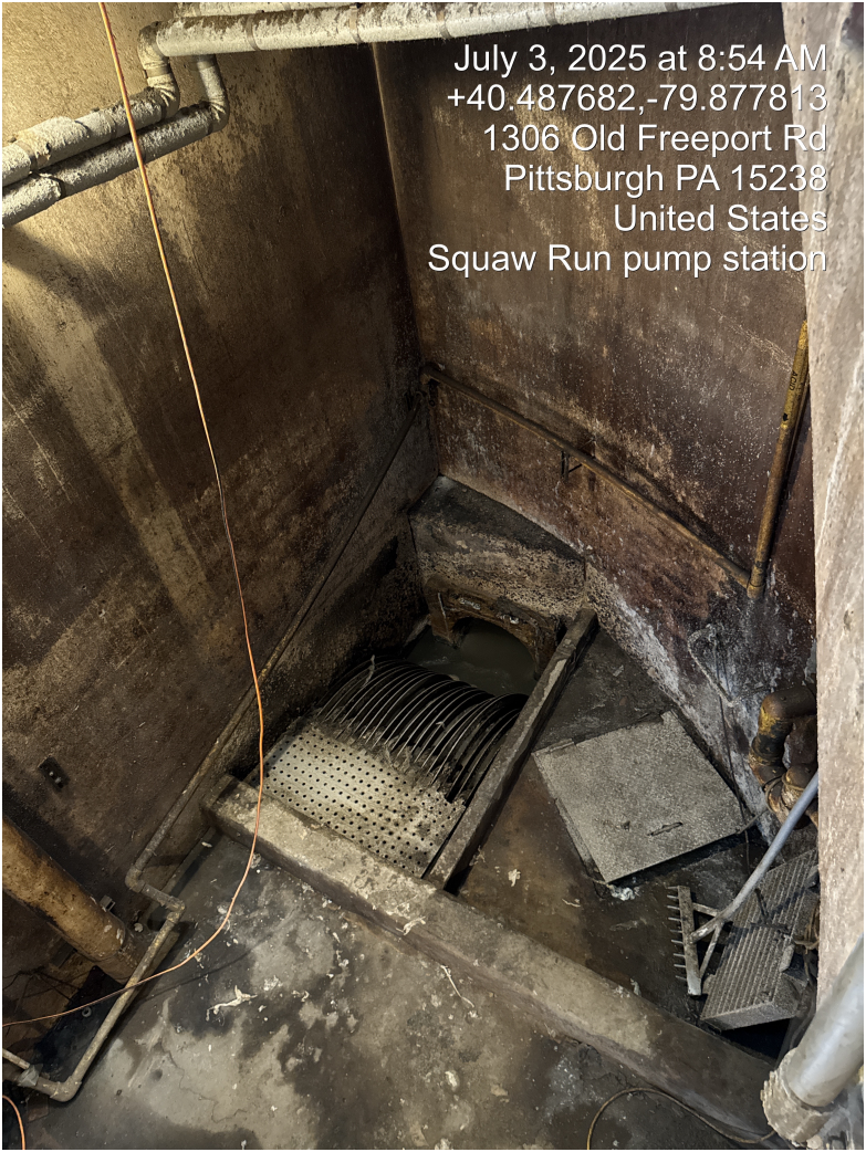
July 3, 2025 at 8:53 AM +40.487790,-79.877908 1306 Old Freeport Rd Pittsburgh PA 15238 United States Squaw Run pump station
