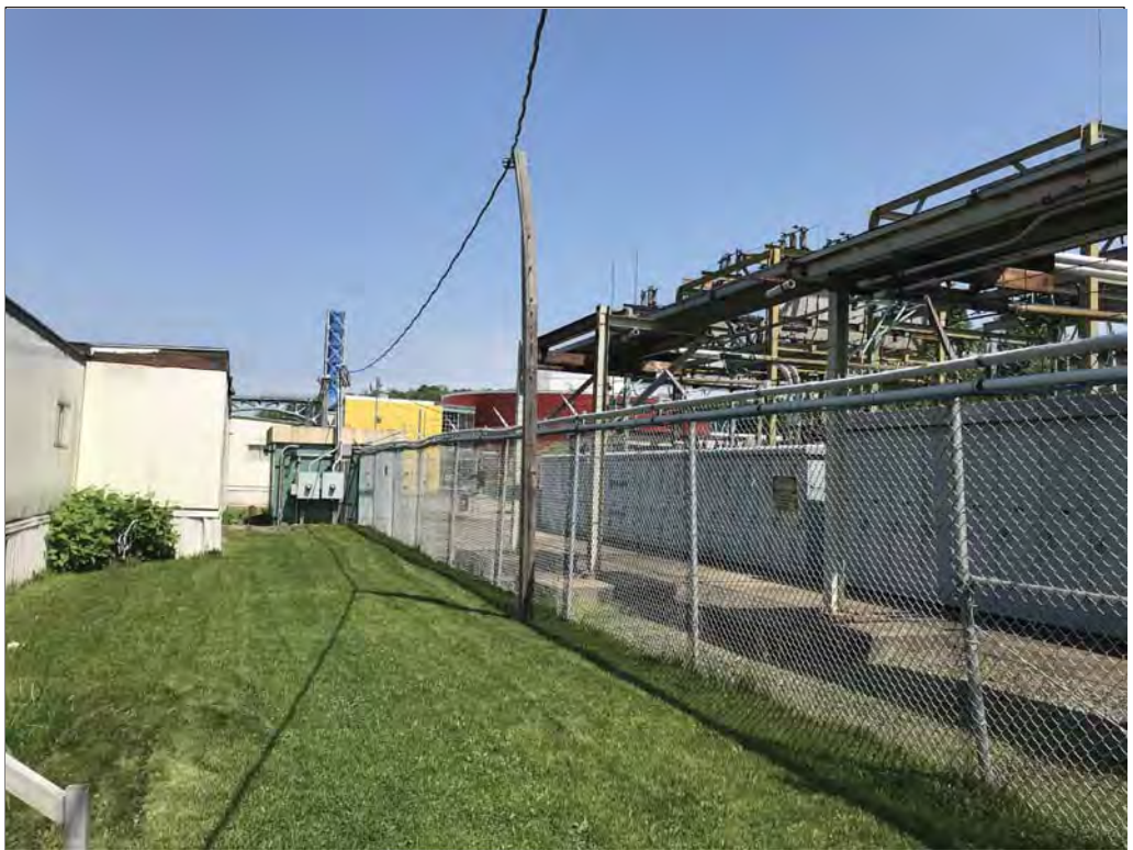
WEST VIEW - EXISTING 5KV SUBSTATION PHOTO 3
