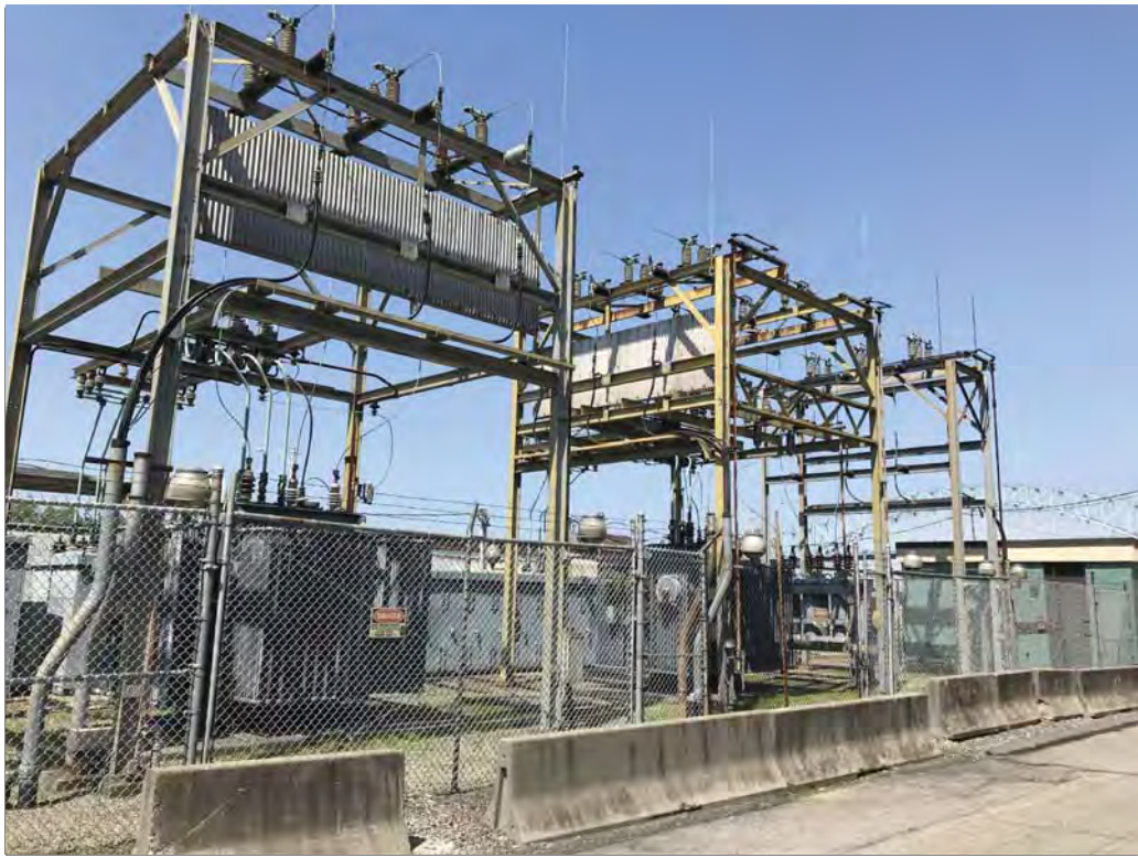
EAST VIEW - EXISTING 5KV SUBSTATION PHOTO 1
