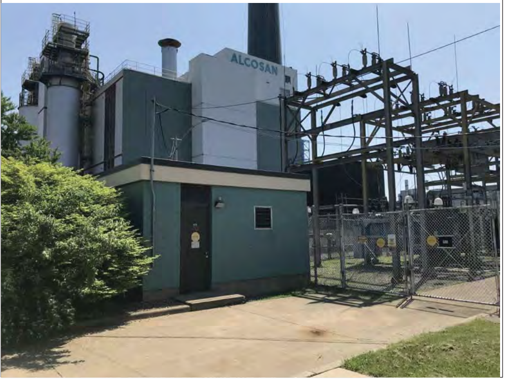
DLC CONTROL HOUSE PHOTO 4
