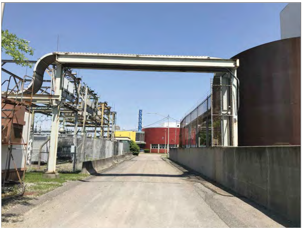
OVERHEAD CABLE TRAY PHOTO 2
