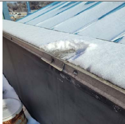
HA #03, Adhesive on Roof Wall Cap Fasteners
