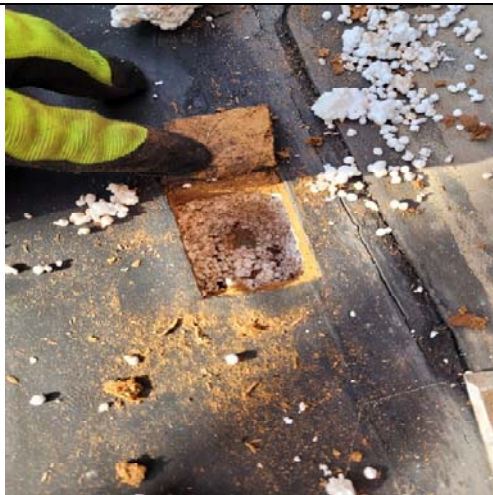
HA #02, Adhesive on Roof
