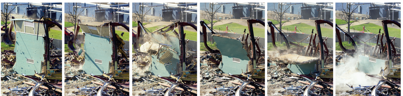
Yielding to plant expansion, the last wall of ALCOSAN's original Operations and Maintenance facility fell on October 8, 2018.
