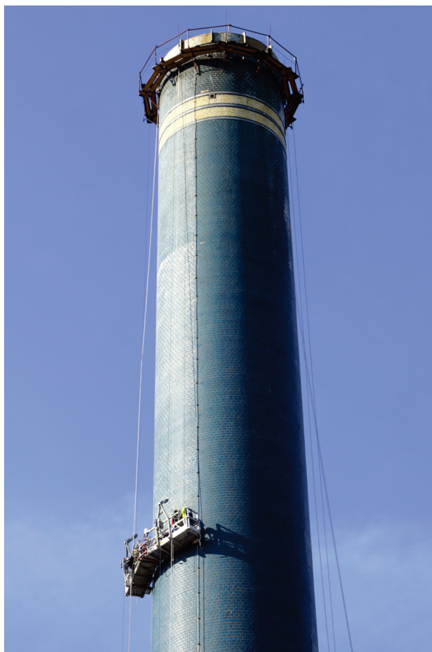
Contractors work from a suspended scaffold platform while completing restoration work on ALCOSAN's 300-foot incinerator chimney.
