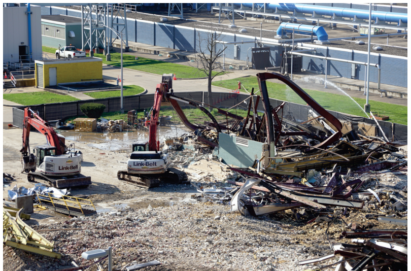
Demolition of the old Operations & Maintenance facility will provide the footprint for expansion of the plant's pumping, headworks and primary treatment capacity.
