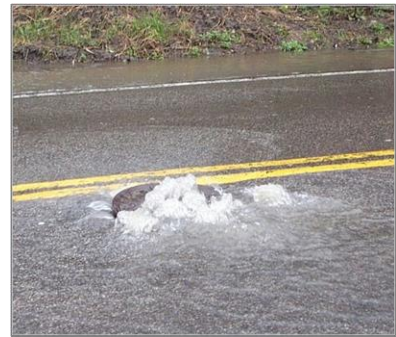
Figure 10-77: Sanitary Sewer Overflow Caused by Excessive Inflow and Infiltration
