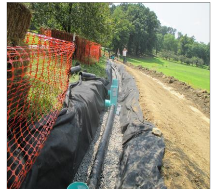
Figure 10-78: Infiltration trenches and berms have been installed to reduce hillside erosion, converting lawns to meadows, and vegetative buffers in Pittsburgh’s Schenley Park.
