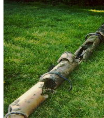
Figure 10-73: Deteriorated Building Lateral Sewer
