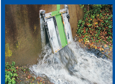
Combined Sewer Overflow (CSO)
