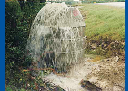
A Sanitary Sewer Overflow (SSO) occurs when a line designed to carry only sewage becomes overloaded with stormwater. This causes untreated sewage to overflow from manholes or back up into basements.
