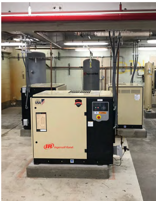
Installation work for the new centralized instrument air system was completed by ALCOSAN's in-house maintenance personnel.
