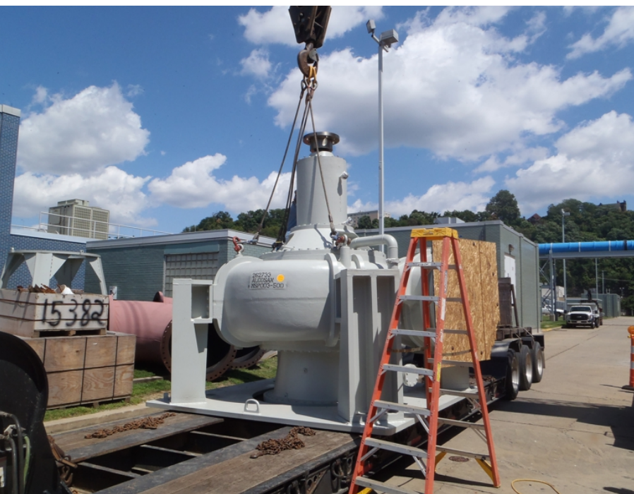
Upgrades to the main pump station included installation of six new pumps, replaced one at a time to maintain operations
