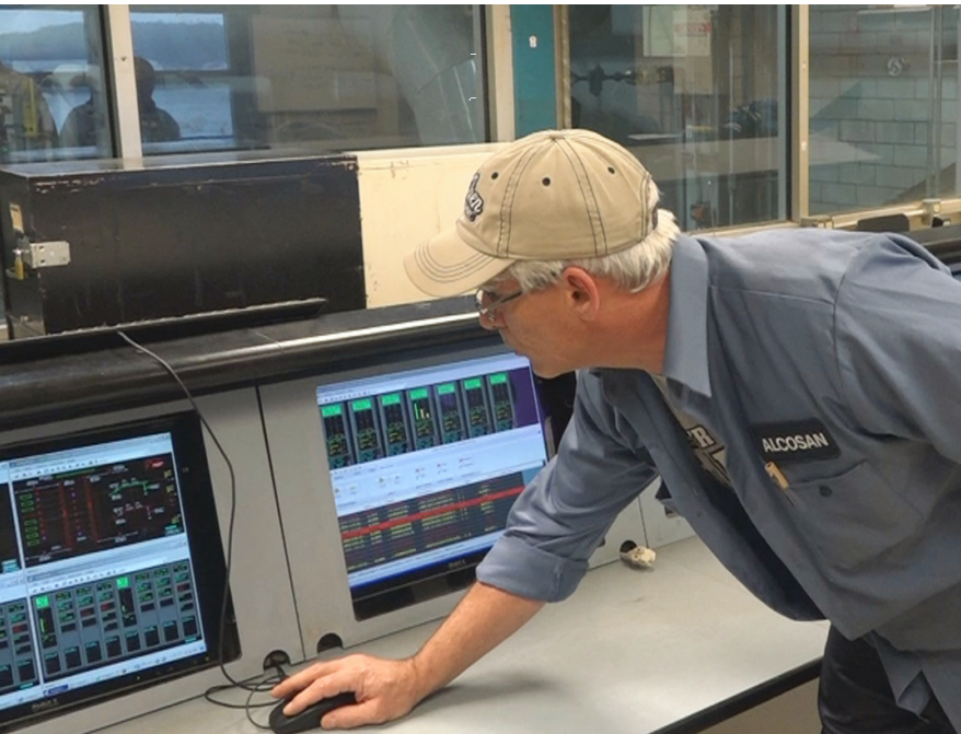
ALCOSAN operators use a distributed control system to monitor treatment processes and maintain an average daily flow of 195 million gallons
